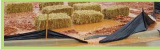
Failed silt fencing and hay bales
